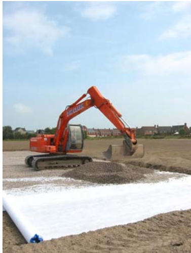
Levelling of base layer over an artificial membrane during construction of cricket wicket for North Somerset Council at Weston Super-Mare.
