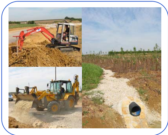
Various stages of road side drainage at Carterton, for Hope and Clay Construction
