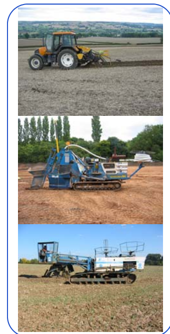
From the top: installing water pipe with the AFT 100, one of our laser guided Mastenbroek 1012 and large scale agricultural drainage with the BT6.
