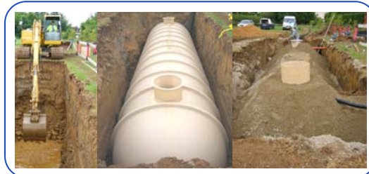
Excavation, installation and back filling of Cess Pit at Shennington Air Field.
