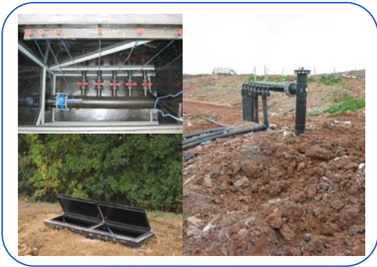
Above and below ground gas manifolds installed and ready for pressure testing at Poplars and Roxwell landfill sites.
